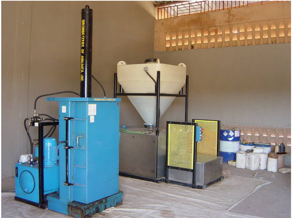
The FAO container washing and crushing system situated outside Bamako.
